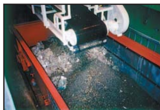
Roll-Off Dewatering Screenings & Grit
